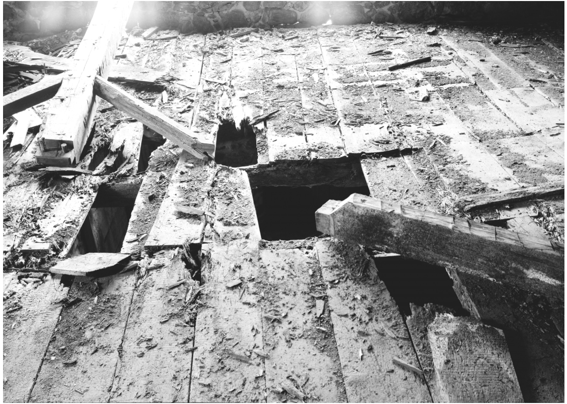
Fig. 20 Collapse of framing and flooring perhaps attributable to poor condition of the roof membrane. (HABS Photograph by Jack E. Boucher, August 1963)
