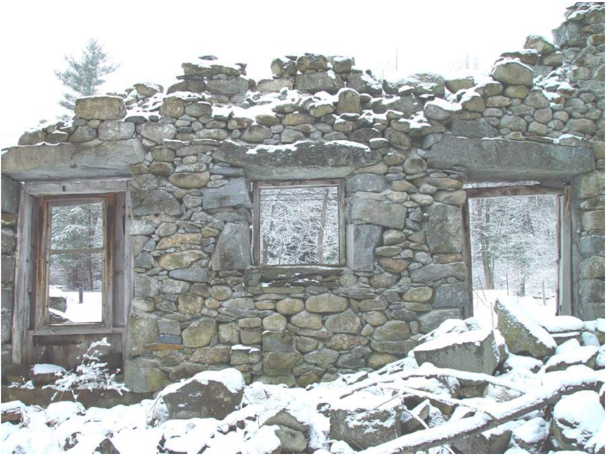
Fig. 26 Snow sitting atop unprotected masonry head and collar joints.
