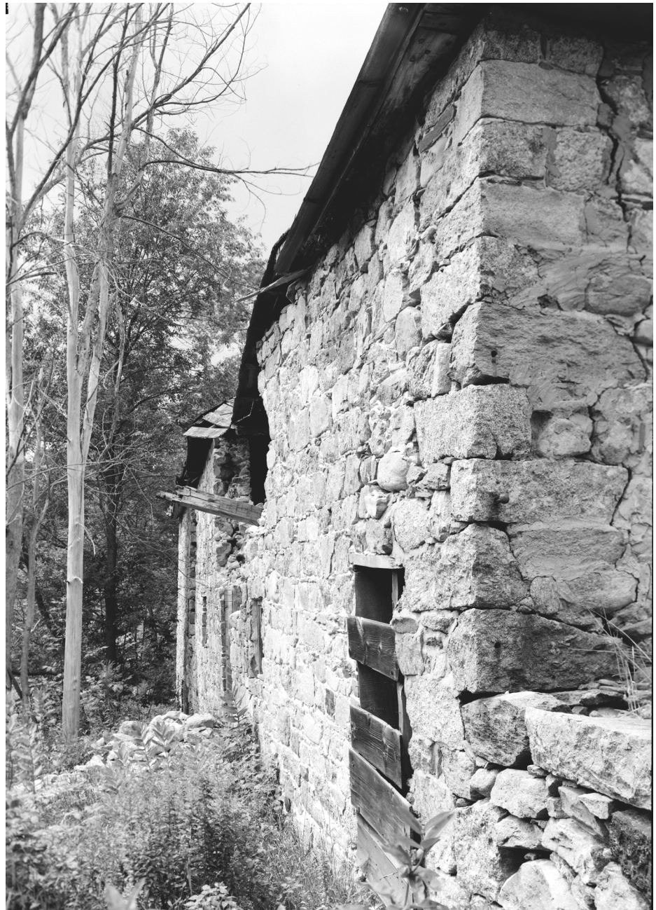
Fig. 22 Breach in south wall stone masonry, and developing vertical cracks at southeast corner. (HABS Photograph by Jack E. Boucher, August 1963)
