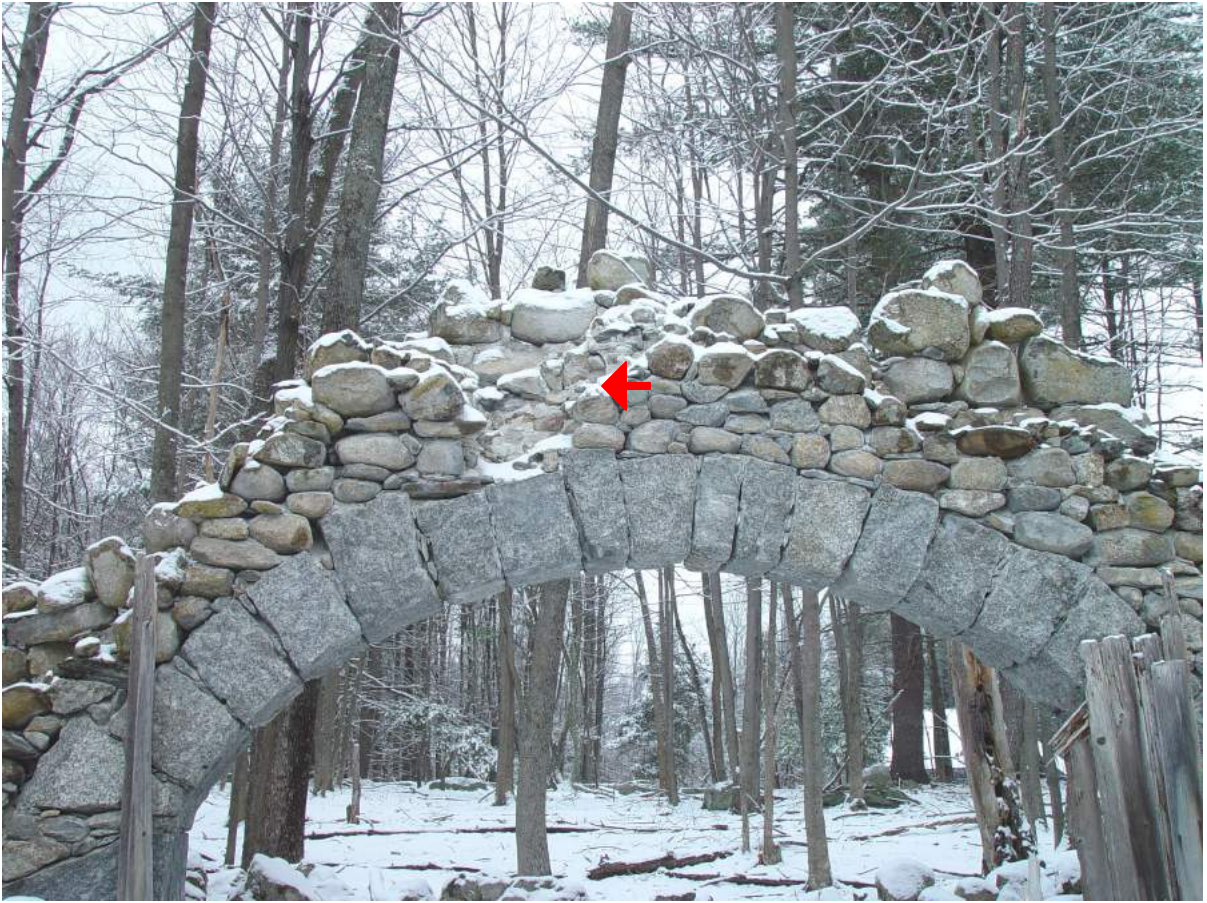
Fig. 23 Recent collapse of masonry above north arch, occurring early in 2004.
