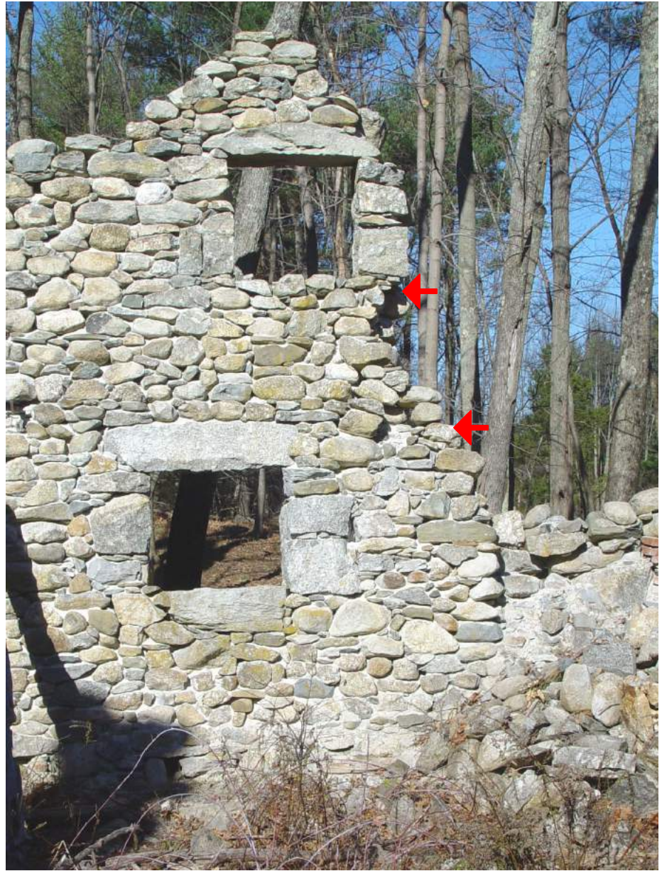
Fig. 32 Instability of second story window jamb caused by loss of inner wythes below.
