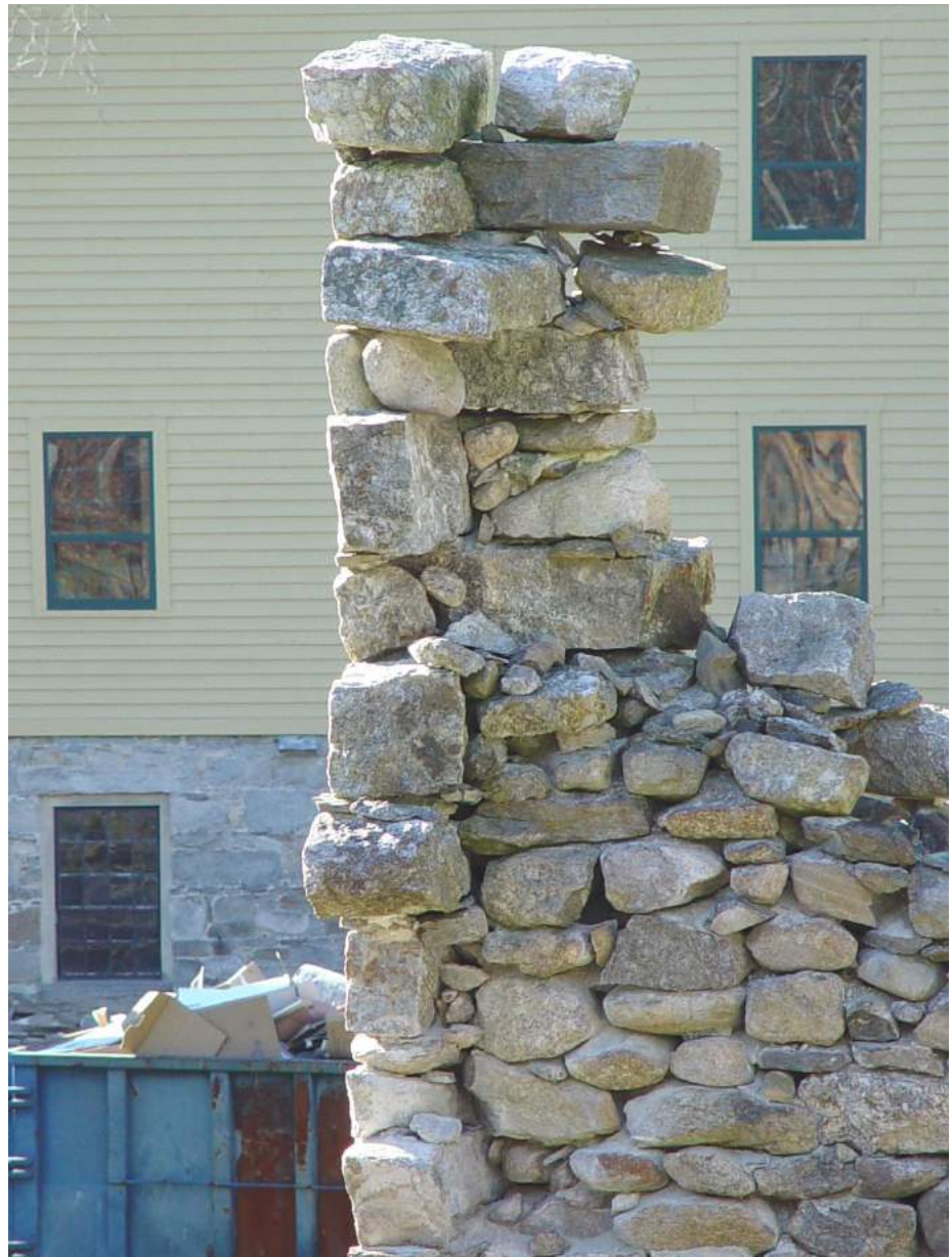
Fig. 31 Top of southwest corner, showing loss of inner wythe.
