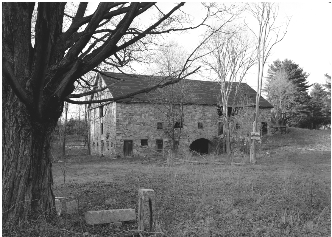
Fig. 19 South elevation showing worsened condition of roof and stone masonry. (HABS Photograph by Jack E. Boucher, April 1963)
