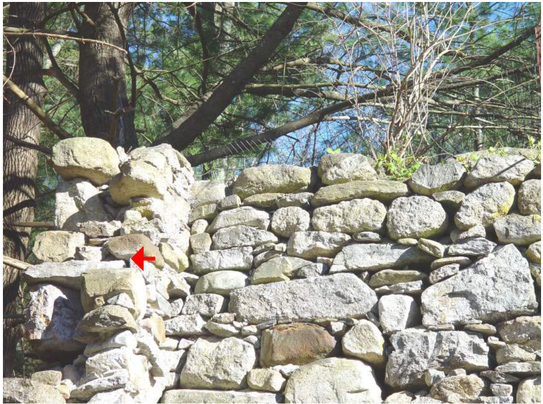
Fig. 4 Cross section of wall showing chinked collar joints, and random headers tying inner and outer wythes.
