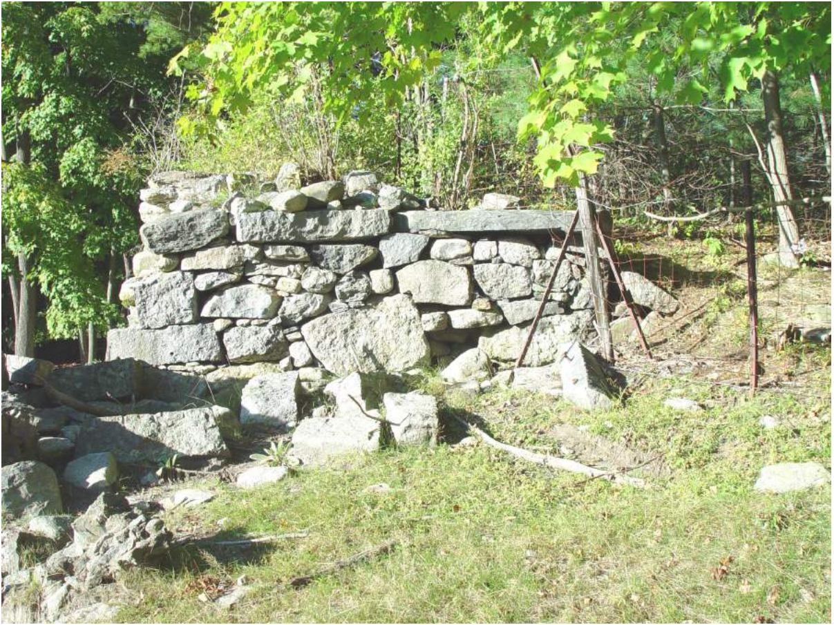
Fig. 36 Dislodging of copings on cheek wall of easterly ramp exacerbated by vegetation growth.
